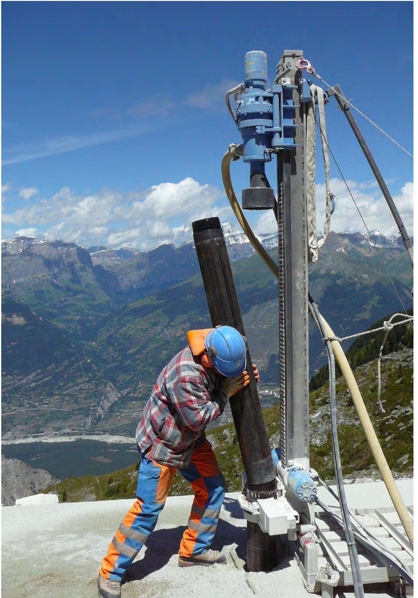
Mounty 92H, diameter 216 mm, length 40 m, test drilling by the dam Illsee, Leuk, Switzerland
